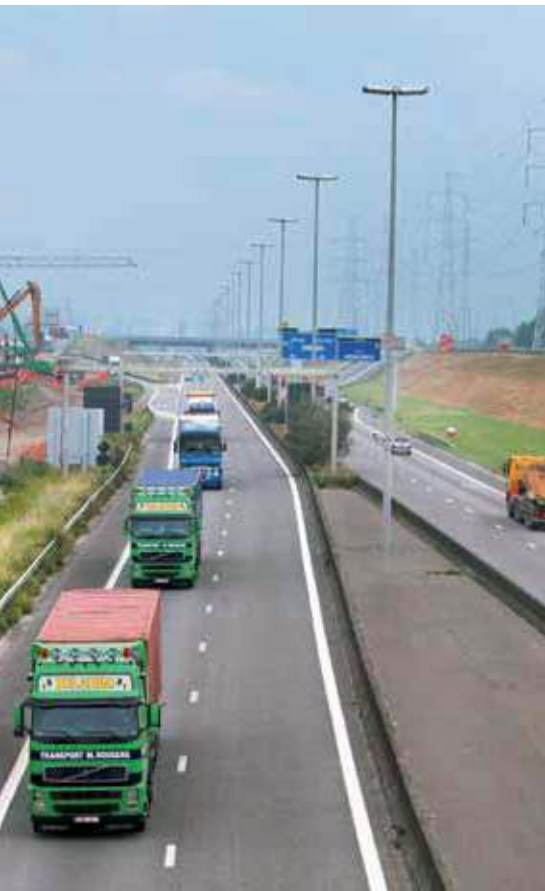
01 Although the volume of work that remains to be carried out on the right bank is less than that on the left bank, its execution is more difficult due to the geological conditions and the narrowness of the site.
