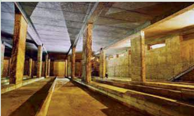
Stade de France (France) – 1998 – Soletanche Bachy Diaphragm walls and barrettes for the La Plaine stormwater basin and P2 underground car park beneath the training ground.
