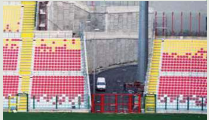
Messina (Italy) – 2001 – Terre Armee Reinforced Earth® diaphragm walls at the Messina stadium, a design whose construction methods and architecture were inspired by the amphitheatres of antiquity.
