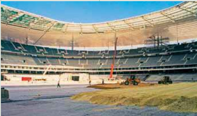
Stade de France (France) – 1998 – Menard Site remediation using a variation of the Menard Vacuum atmospheric consolidation process. The system remains in use to this day: accumulated hydrocarbons are regularly pumped out.
